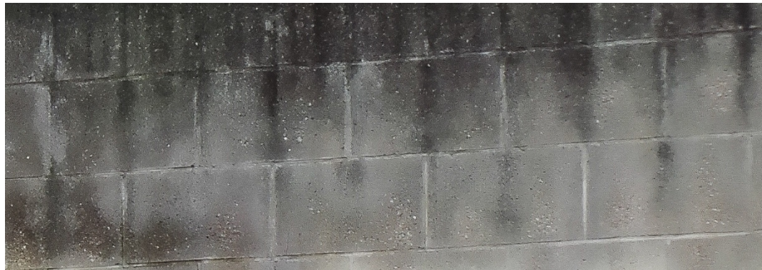
Mold on wall
