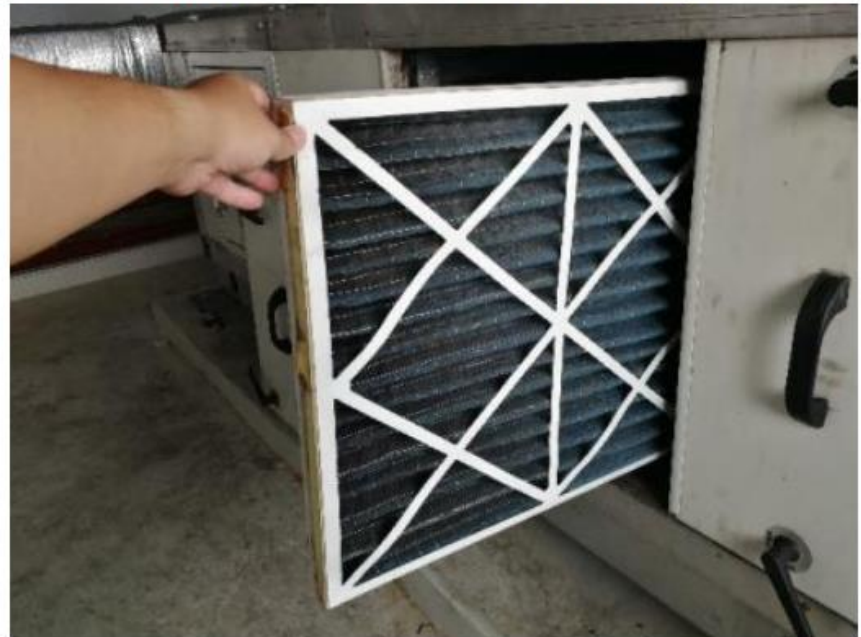
Checking air handling unit pre-filter
