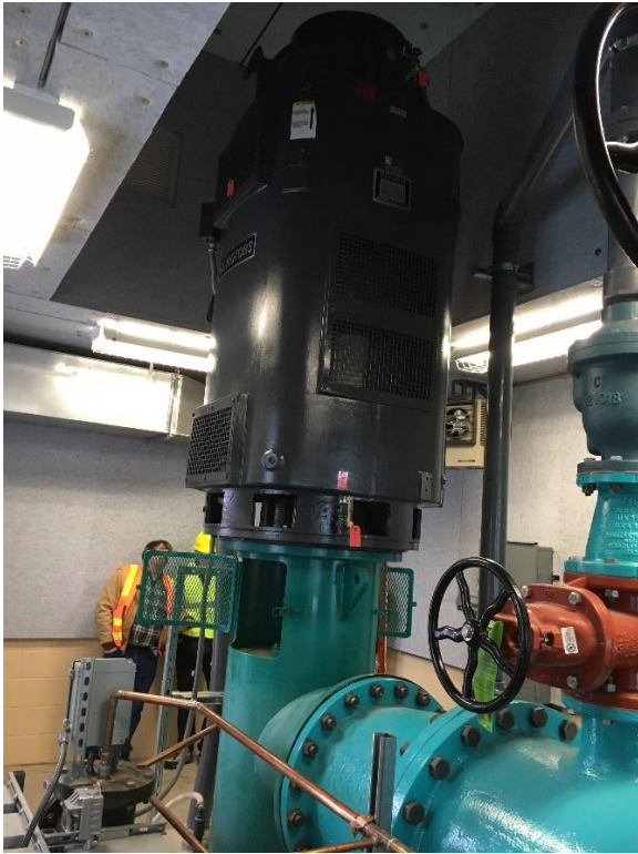
New pump motor at Central Well 2.
