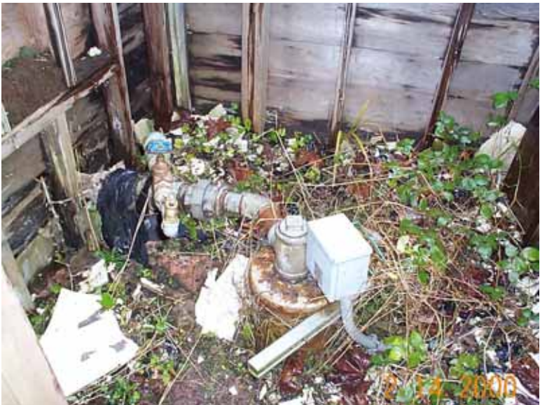
Poor housekeeping of the well house
