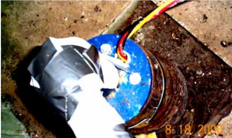
Opening in well casing and no screened vent
