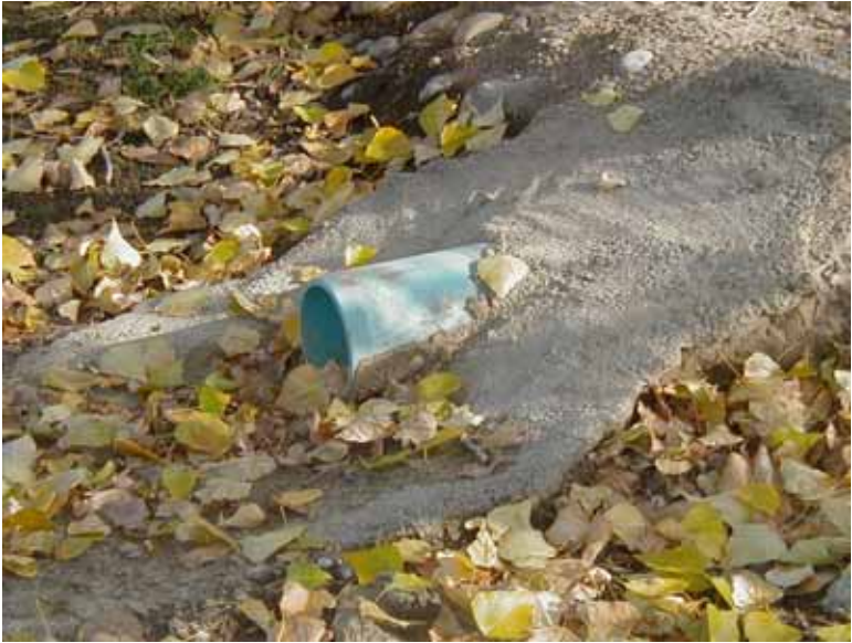
Unscreened reservoir overflow
