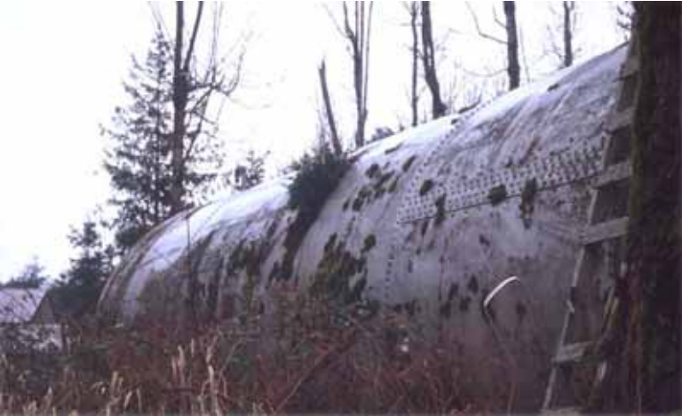
Poorly maintained storage tank with ferns sprouting from top
