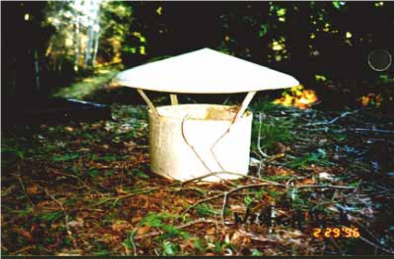
Unscreened storage tank vent
