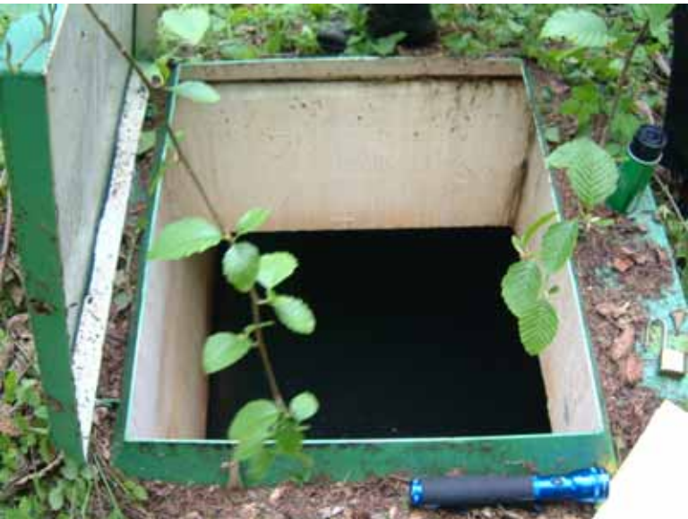
No gasket seal on the storage hatch cover
