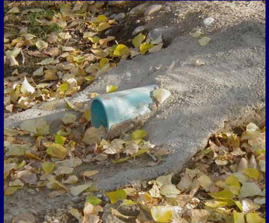
Unscreened Reservoir Overflow.
