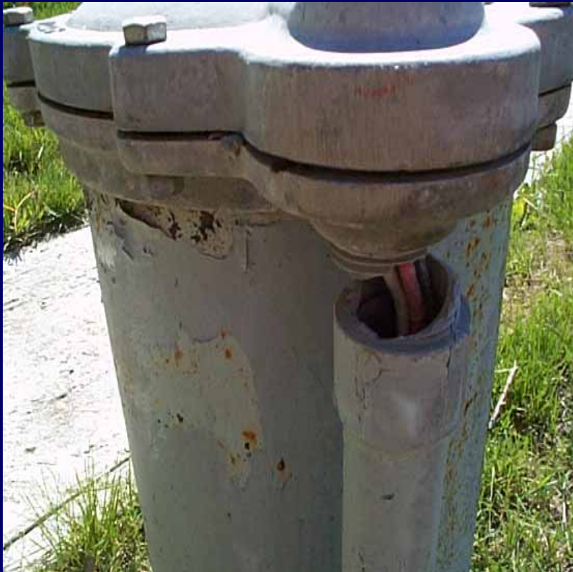
Conduit separated from Well Cap.
