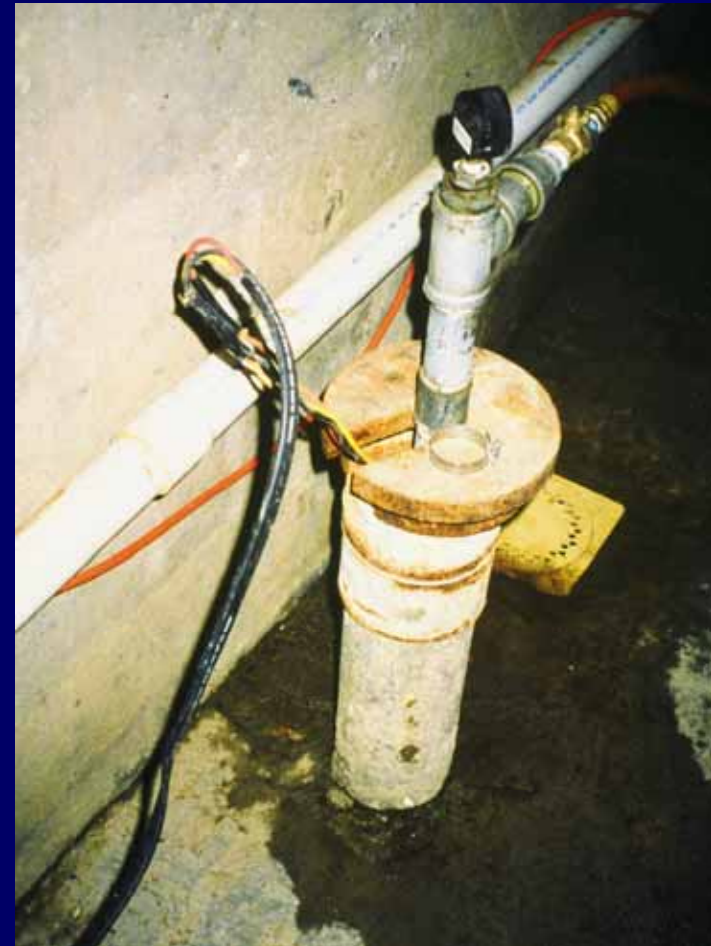
Lack of screened vent and holes in Well Cap.
