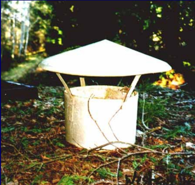
Unscreened Reservoir Vent.
