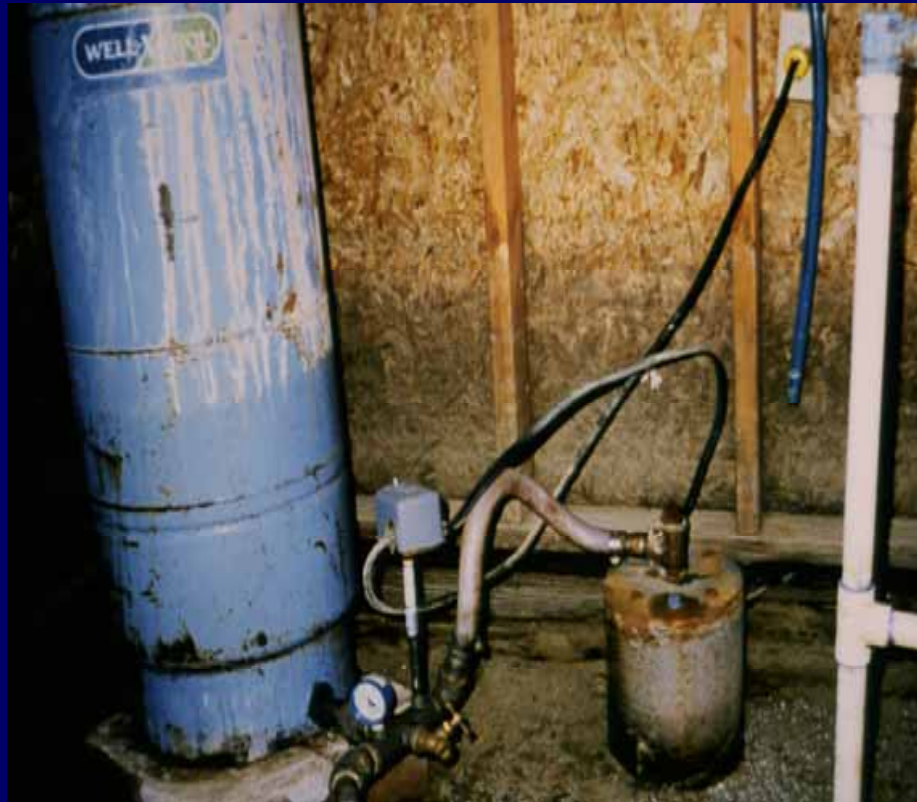
Flooding at Well Head.
