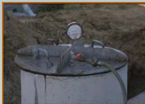
A tank is sealed and placed under negative air pressure. It's considered water-tight if no pressure loss is recorded within 5 minutes.
