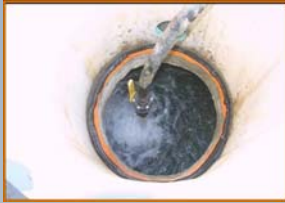
A tank is filled with water. If there's no measurable water loss within one hour, it's considered water-tight.
