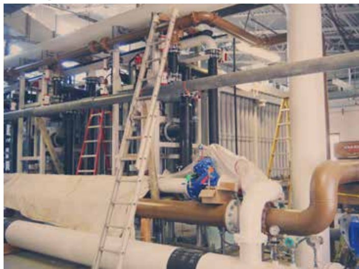
New membrane plant under construction in Port Townsend. Photo courtesy Janet Cherry.
