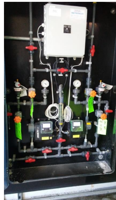
New chlorination system controls
